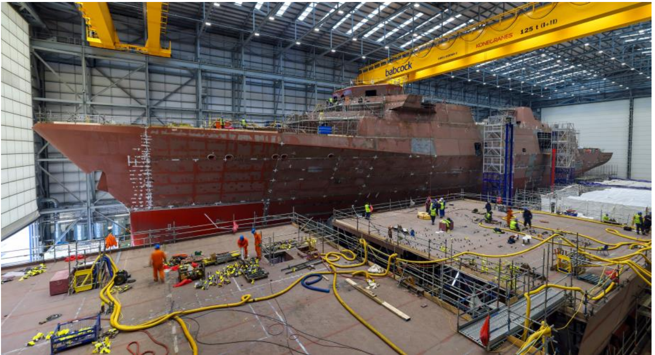
Figure 10. HMS VENTURER (Type 31 Frigate Ship 1) and HMS ACTIVE (Ship 2) in build in Rosyth, Scotland (photo taken April 2024).
