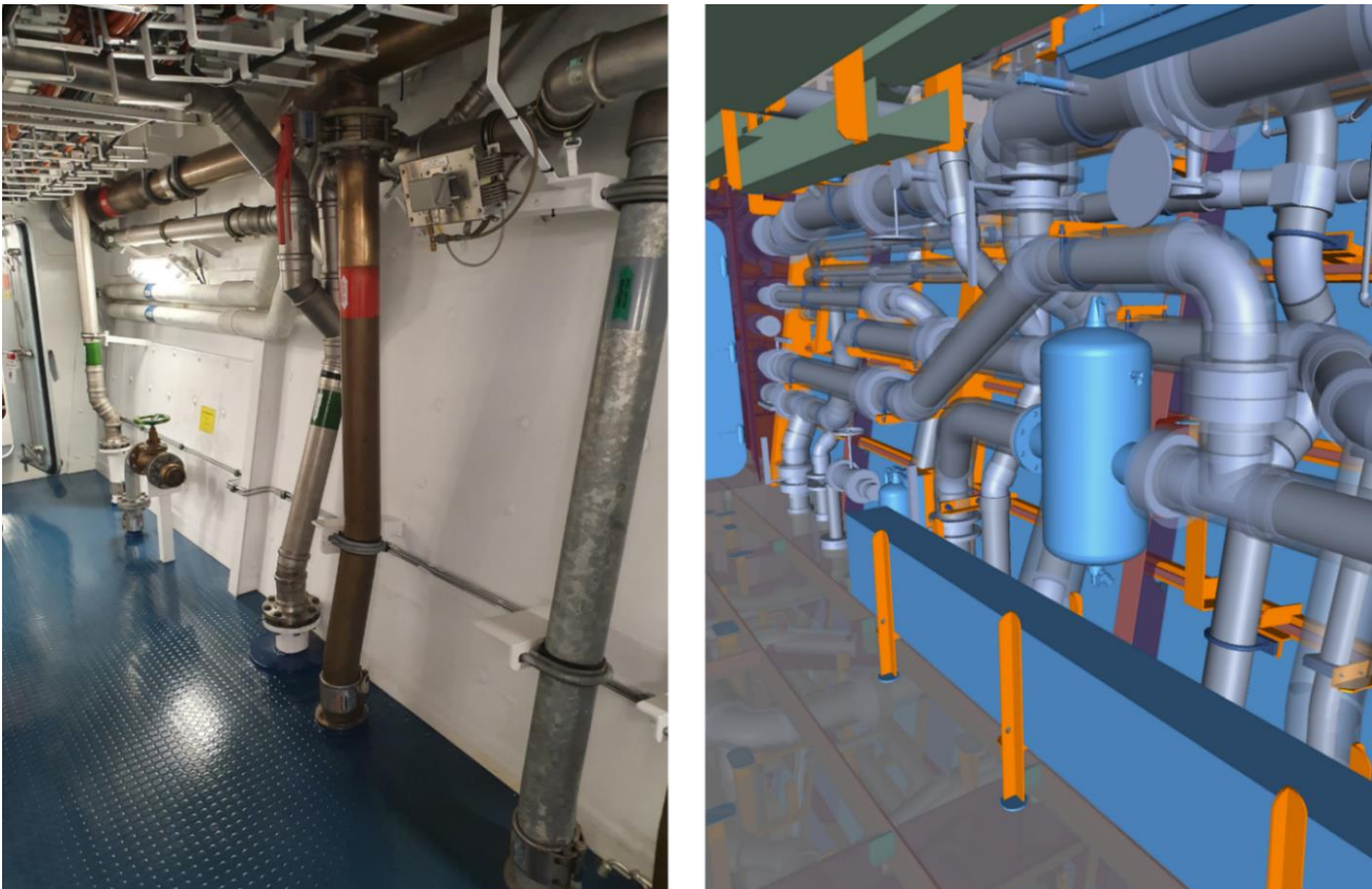
Figure 7. Example of complexity introduced by alternate regulations and standards, supporting recoverability actions. (image left) 'Parent' class passageway; (image right) the equivalent location in Type 31 (extracted from the Type 31 3D detail design model).
